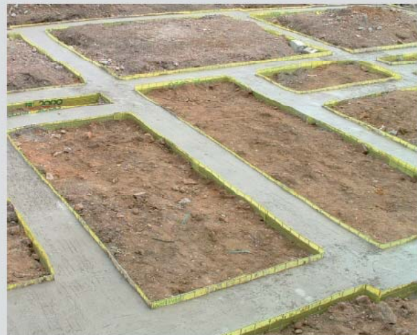
Finished ground beams ready for the next stage of the build process.
